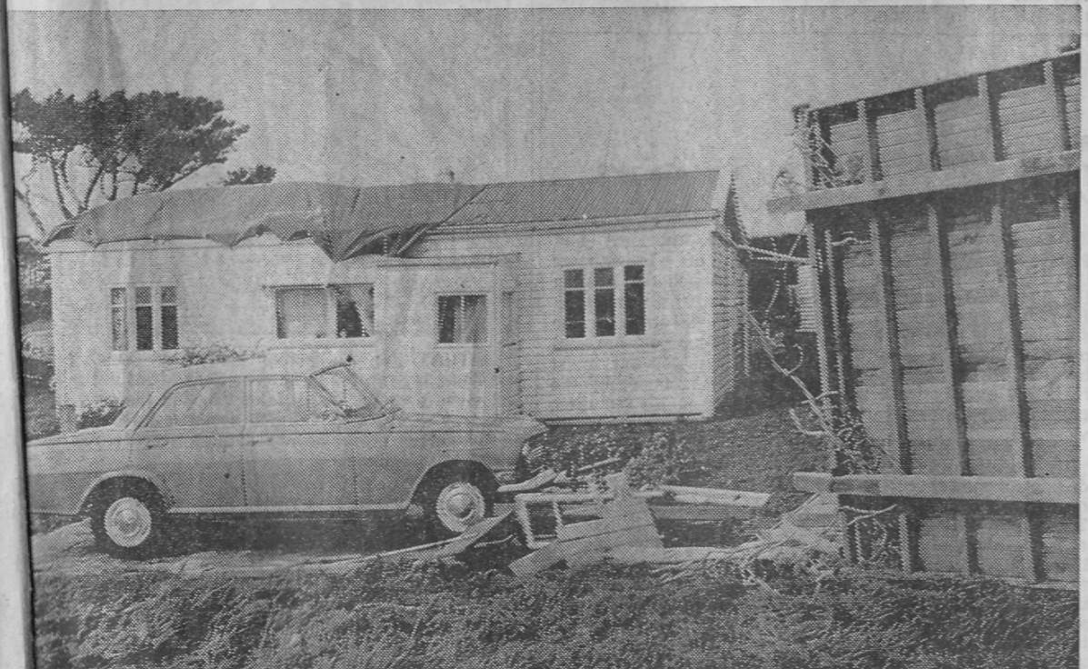
Furness' partially de-roofed cottage on the Armstrong property in Waitetika Rd. The garage was lifted off its foundations and dumped (right) without scratching the cars.
